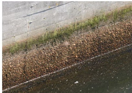
Fig. 8.8.1: Heavy leaching and damage to the structural concrete are observed particularly in the water splash zone of biological treatment basins.
