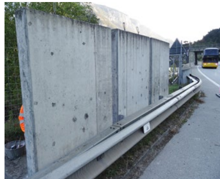
Fig. 8.2.4: Potential measurement on a retaining wall along a road with heavy traffic with high use of de-icing salt, after less than 10 years of exposure. The darker the coloration, the higher the potential for corrosion.
