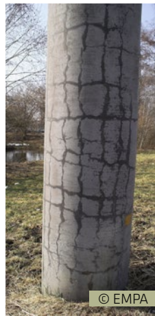
Fig. 8.6.3: The appearance of ASR damage can be assessed very well on the drying concrete surface of this bridge pylon. Damage can appear within years or only after decades.
