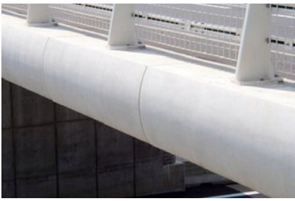
Fig. 8.9.4: Highly stressed building components such as columns and beams are made of high strength concrete. High resistance to external influences also makes high strength concrete an ideal protective coating for exposed construction elements.
