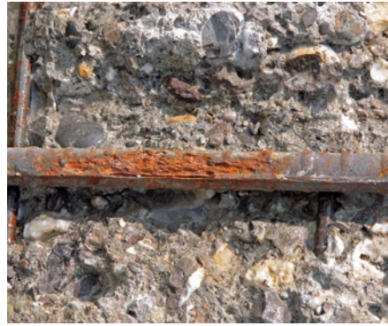
Fig. 8.2.1: Damage to concrete structure due to insufficient concrete cover and low concrete quality
