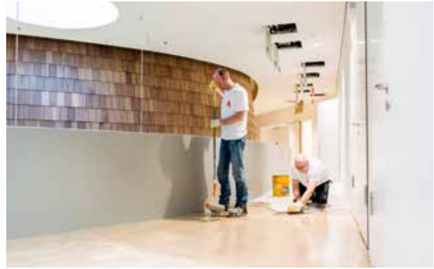
STEP 2. A liquid primer is applied to assure good bonding of the flooring, which is typically done by trowel and roller. The adequate method can be selected depending on the quality of the subfloor.
