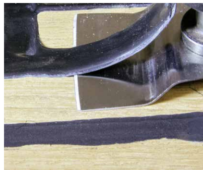
Fig. 49 Picture Removal overstanding Sikaflex®-290 DC PRO with a vibrating scraper power tool
