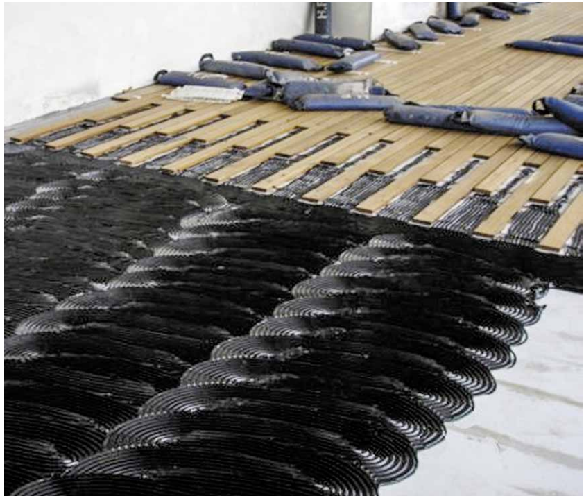
Fig. 14 A teak floor being laid, showing the bedding compound and the weights to hold it in place
